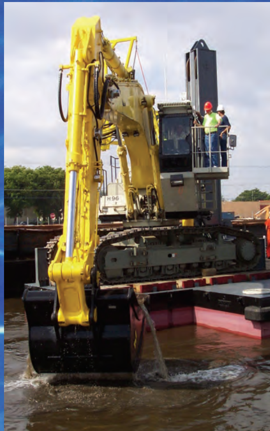
ABOVE PHOTO: Miami River Maintenance Dredging and Environmental Cleanup project in action.
